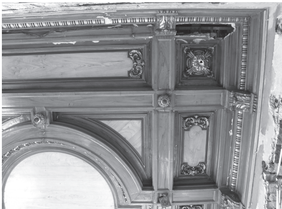
Fig. 12. Detaliu de plafon repictat, imitație lambriu de lemn necaracteristic perioadei / Detail of the repainted ceiling, not typical imitation of wood paneling Sursa / Source: Arhivă personală / Personal archive
